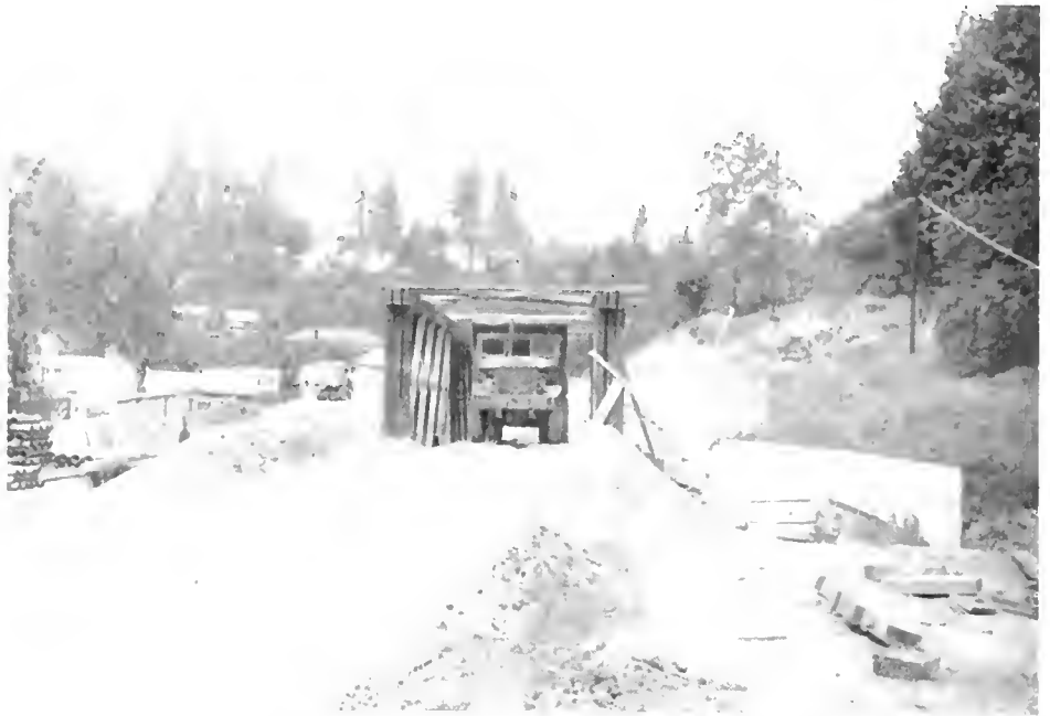
This photograph shows the Camino, Placerville and Lake Tahoe Railroad truss that was salvaged and used to span a highway grade separation structure to permit the use of over-legal loads during construction
